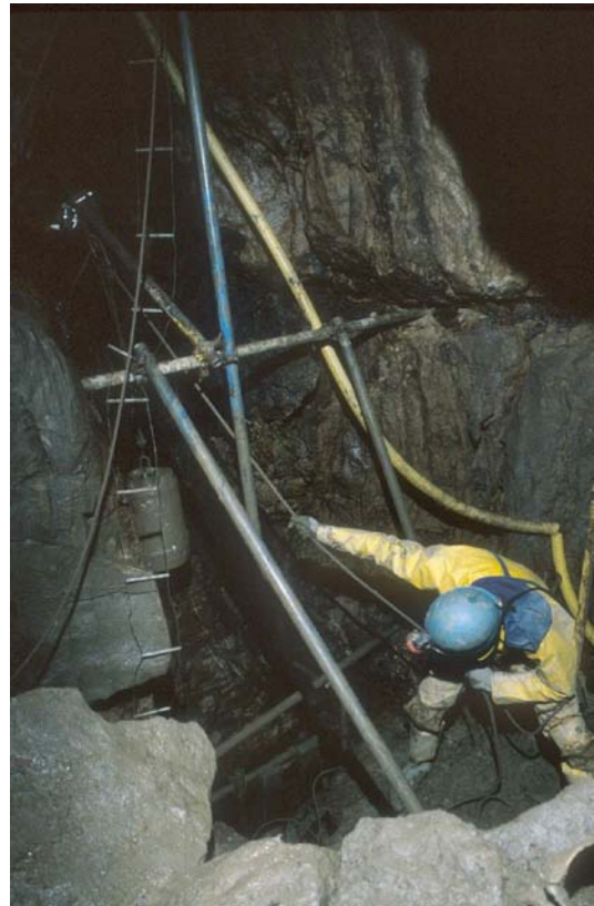
ALISTER HAULS BUCKETS ABOVE THE EXPLORATORY SHAFT AT THE BOTTOM OF SEALEY'S FAULT CHAMBER. DIG LATER ABANDONED.
